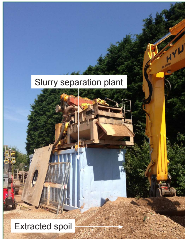
Figure D2: Slurry separation plant (image courtesy of Morgan Sindall)
